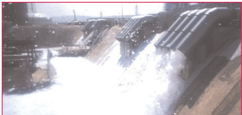
Angus Fire Engineering has designed numerous LNG fire protection systems around the world
